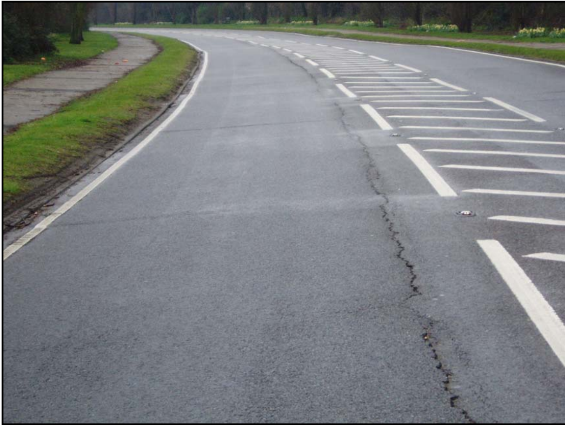
General condition of carriageway before removal of asphalt. Reflective cracking identifies failure of concrete and subgrade layers
